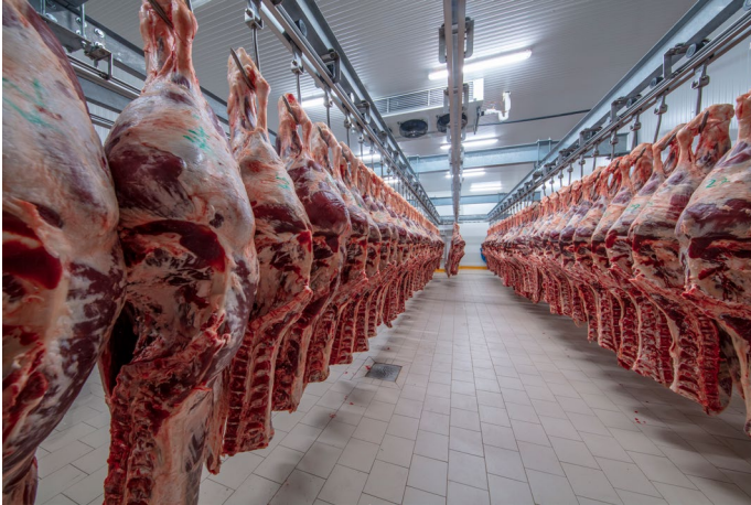
Slabs of beef hang from hooks in a cold storage room. There is a floor drain in the beige tile floor of the room.
